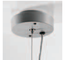
Ceiling rose with power supply cable.
